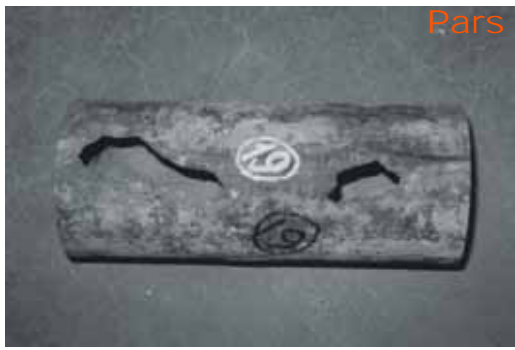
Figure 4. Heavily corroded gray cast iron pipe. (City of Toronto)
